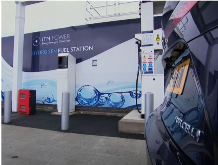
The network of hydrogen fueling stations is slowly growing
