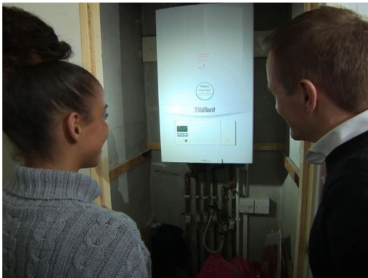
Chloe Edwards-Simpson's boiler could be converted to use hydrogen
